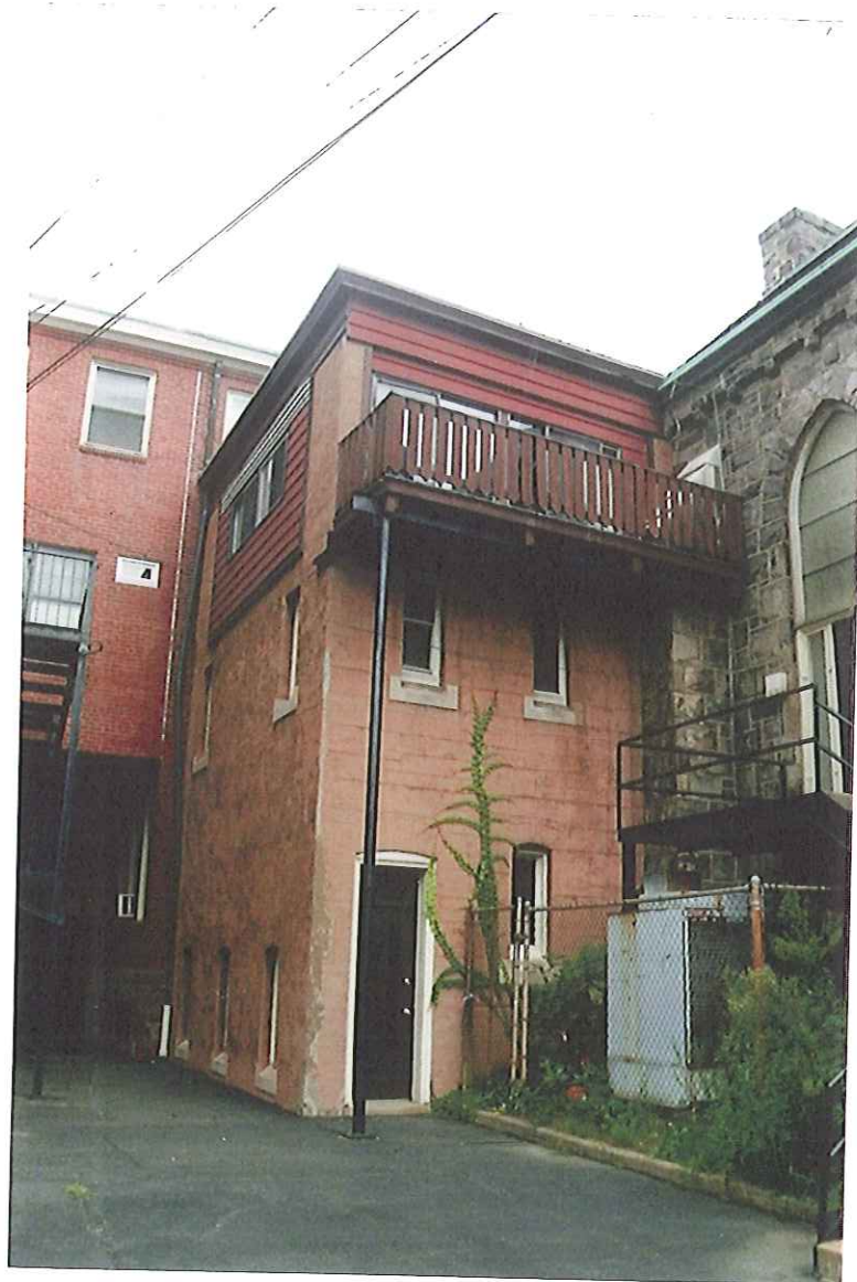
THREE LEVEL APPENDAGE TO CHURCH BUILDING AND ADJOINING SOUTHERLY WALL OF CHURCH AND EASTERLY WALL OF CONVENT
